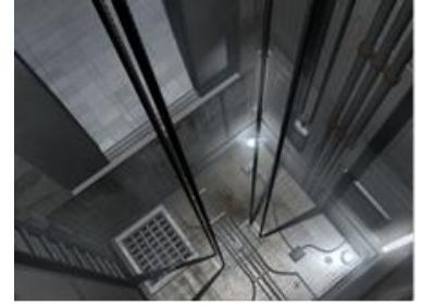
Elevator shaft subject to wind issues
