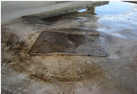
Failing Patch Repair on Roof
